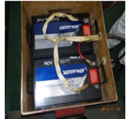
New GMDSS batteries
